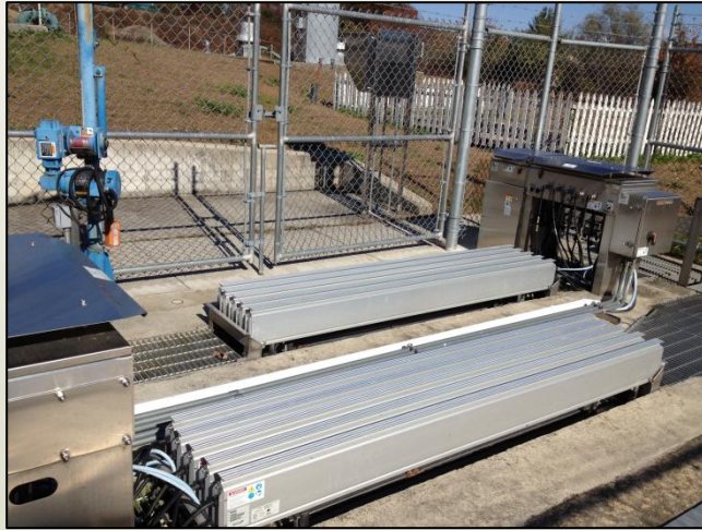
UV Disinfection System
